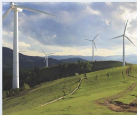
Wind turbine generator
